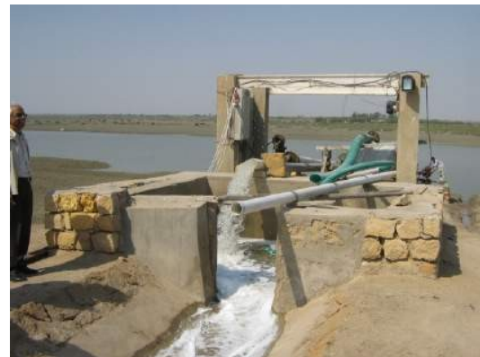
Pumping station at Ghorabari
